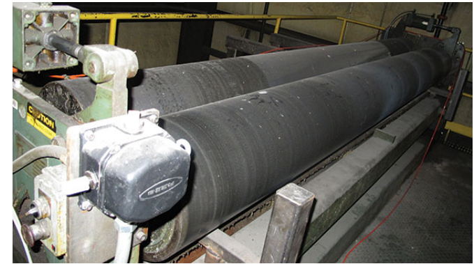
Conveyors & Infeed Rollers
